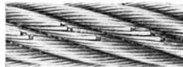
Parallel wear pattern in the cyclical bending area, ending in wire breakage. Caused by grooves in rope sheaves that are too small or too big.
